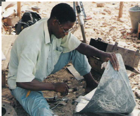
Photo 54. Hammering on the inside of the seam to make it hold tightly.
